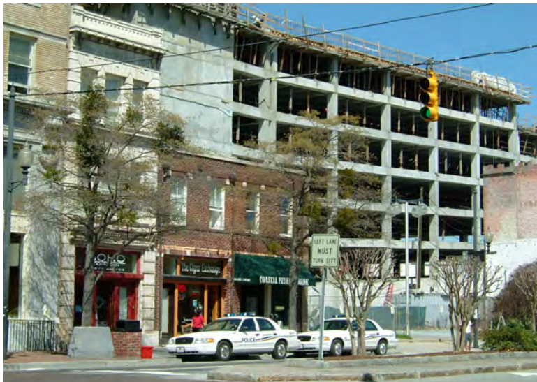
A new parking garage on 2nd Street (shown here under construction in a view from Market Street) opened in Summer 2004.
