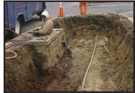
Figure 3-2 Excavation of a landscape island to create a bioretention cell. Source Larry Coffman.
