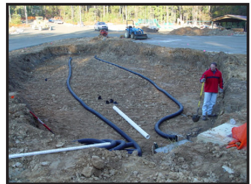
Figure 5-7 Bioretention cell under construction in a parking lot showing underdrains. Source Bill Hunt, NCSU.
