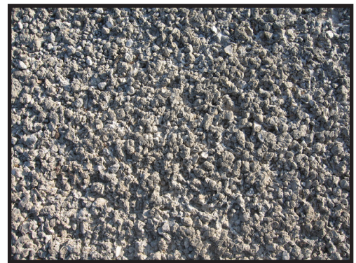
Figure 5-24 Close-up of porous concrete at Costco in Wilmington.
