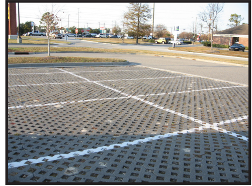
Figure 5-22 Open-celled block pavers within overflow parking area at Best Buy in Wilmington.
