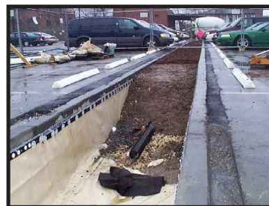
Figure 3-20 Excavation of bioretention cell with concrete and plastic liner at Navy Yard. Source LID Center.
