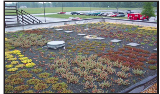
Figure 5-34: Wayne Community College Green Roof in Goldsboro one year after planting (May 2003). Source: NCSU
