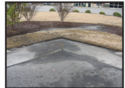
Figure 4-10 Curb cut in Mayfaire in Wilmington, NC. Photo taken after rain event evidencing where water entered the bioretention area.
