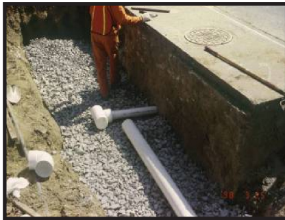
Figure 3-3. Urban retrofit showing construction of underdrain system and gravel infiltration reservoir. Source Larry Coffman.
