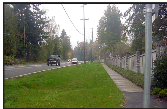
Figure 4-17 Example of a shallow roadside swale system with under drains to facilitate drainage and reduce ponding time. Source, Portland, OR. .
