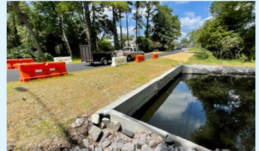
This new bridge on Mallard Street is part of the Clear Run Branch drainage project.
