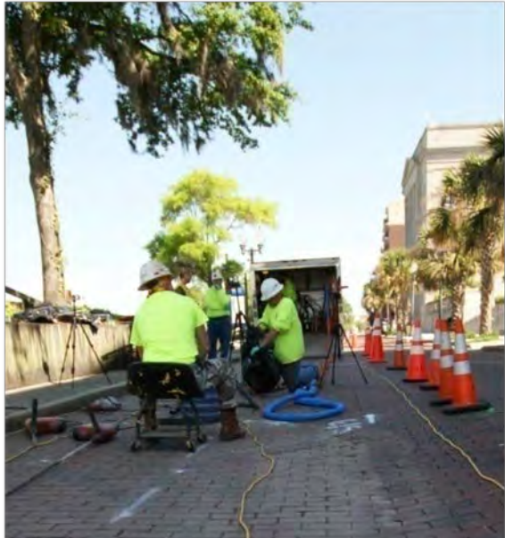
Contractors injected a polymer into the soil to stop erosion of soil through the bulkhead
