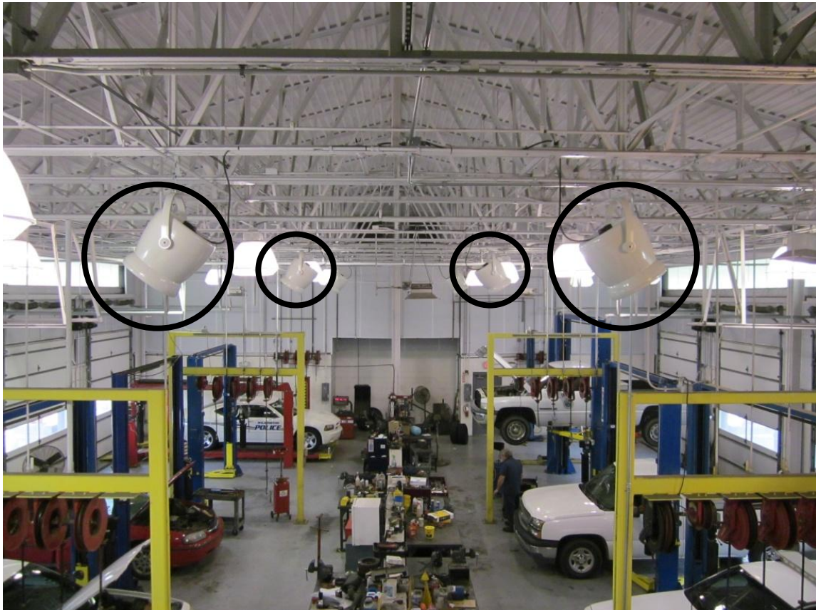
Fans installed in the Fleet Maintenance building as a part of the EECBG grant Photo Source: David Lallier
