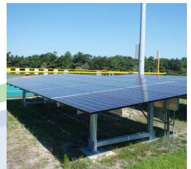
Miracle Field Solar Array at Olsen Park Brax Stadium
