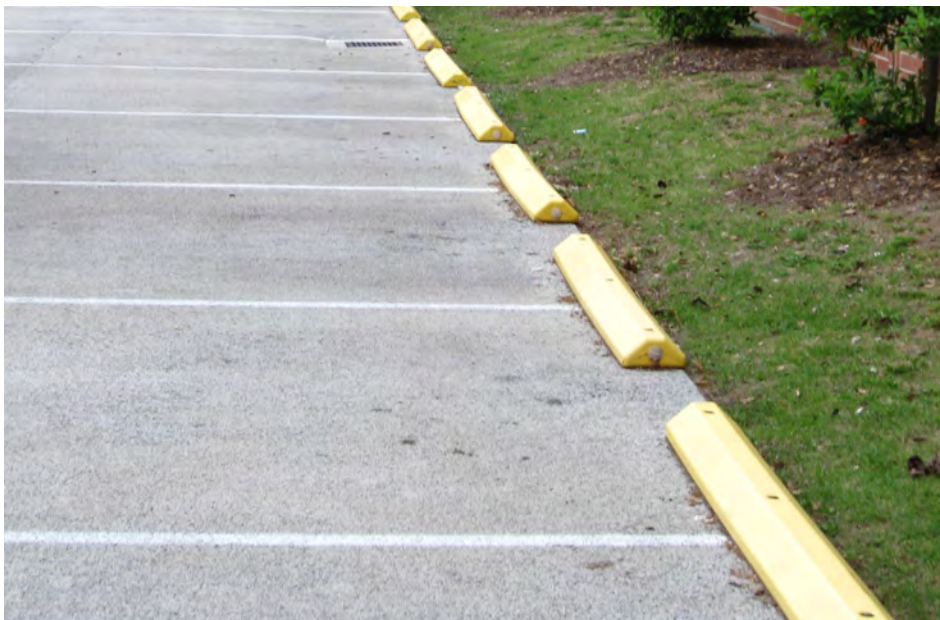
Figure 7. A permeable pavement lot in Wilmington, N.C.
