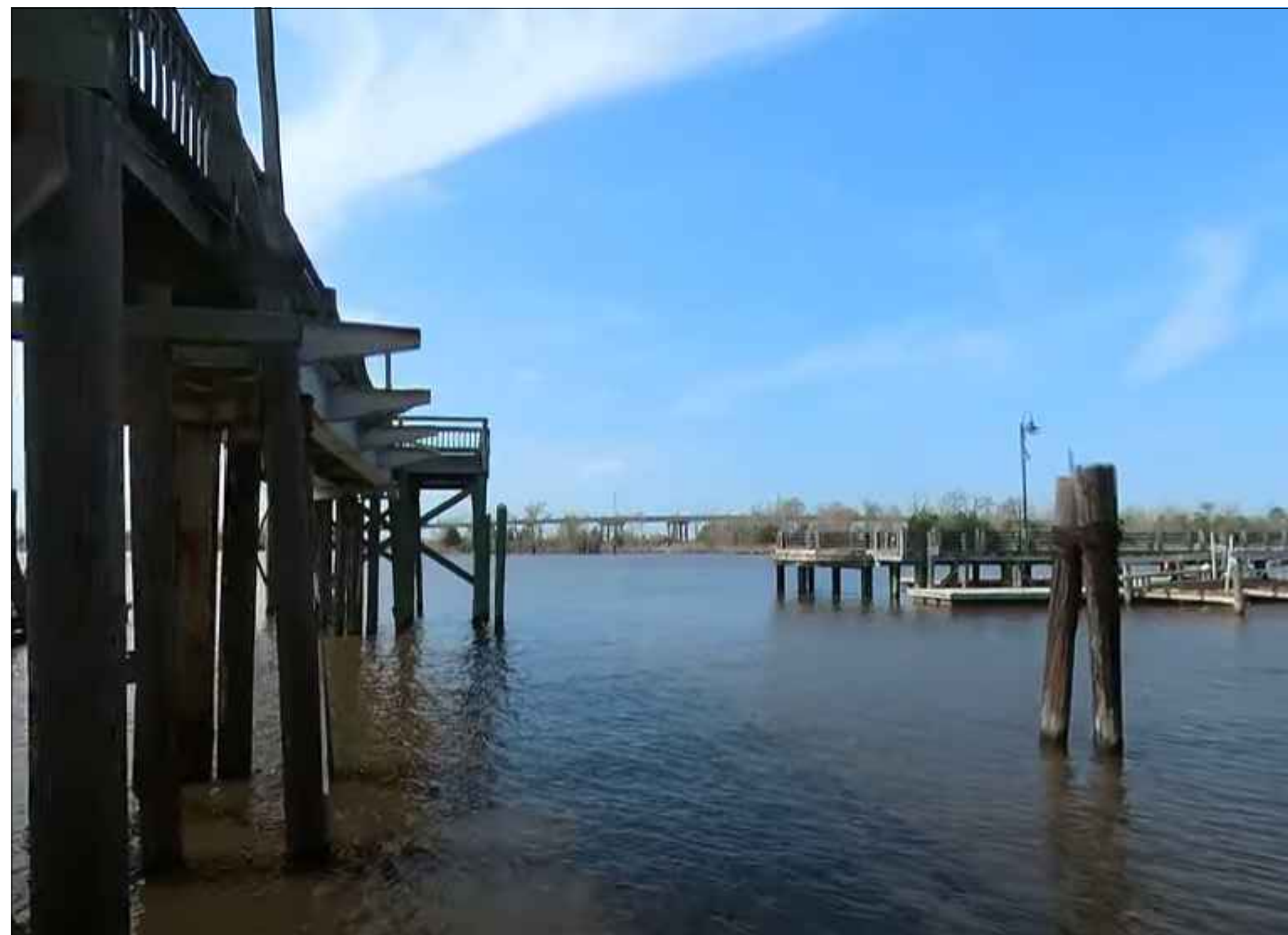
3 MORING DOLPHIN C203
